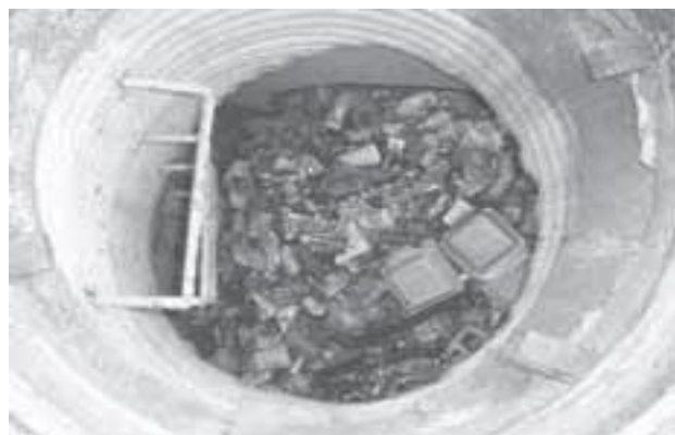
Trash and sediment can quickly accumulate in underground detention facilities requiring frequent clean-outs by professionals.
