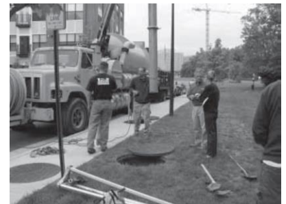
A vacuum truck may be required to remove sediment from stormwater facilities located underground.
